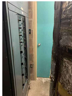
8 PANELBOARD "MDP-M" 2ND FLOOR
