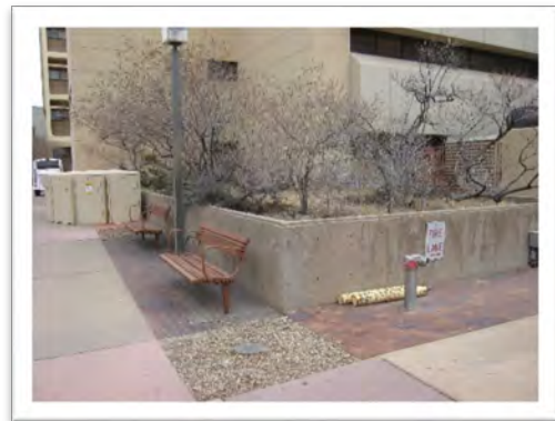
BRF wet pipe fire department connection
