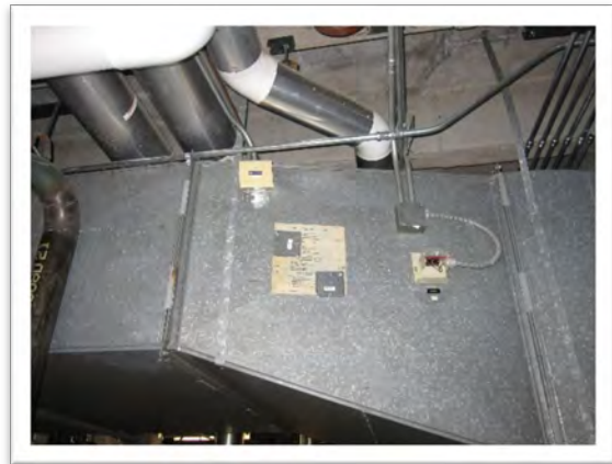
Typical abandoned relay and smoke detector
