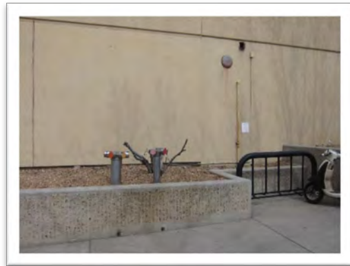
BMSB standpipe and wet pipe connections
