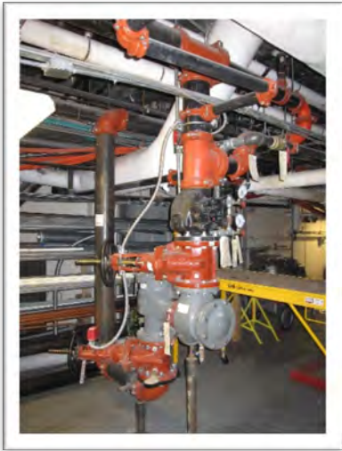
BMSB main fire protection riser
