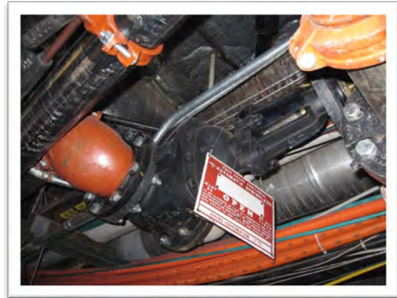
BMSB fire service connection to campus main
