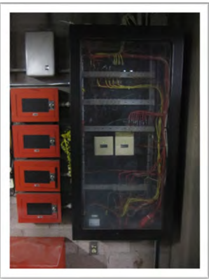
Old BRF FACP now functions as a j-box
