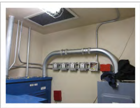
BMSB existing elevator relays
