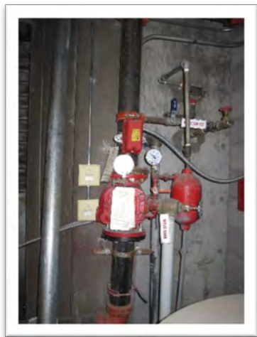
BRF main fire protection riser
