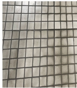
Cracked and uneven flooring
