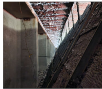
Lack of proper insulation and vapor barrier
