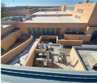
Exterior mechanical, chemical, and electrical rooms
